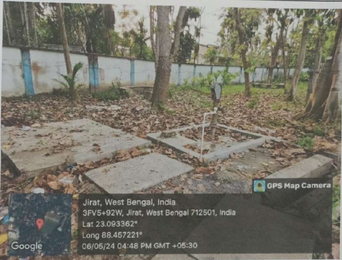
Vertical Filter Chamber With Silt Chamber (2)
