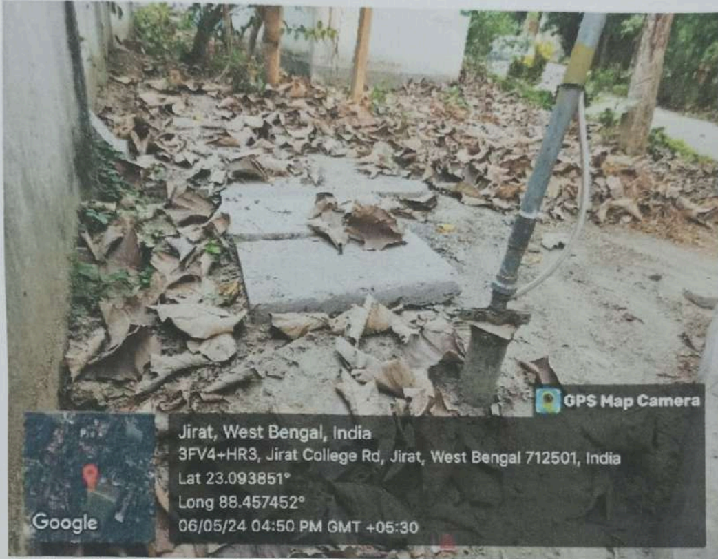
Vertical Filter Chamber With Silt Chamber (3)
