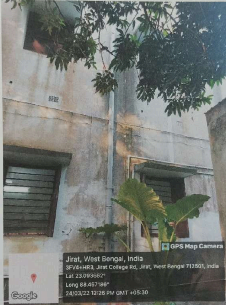
Collection of rainwater from the roof
