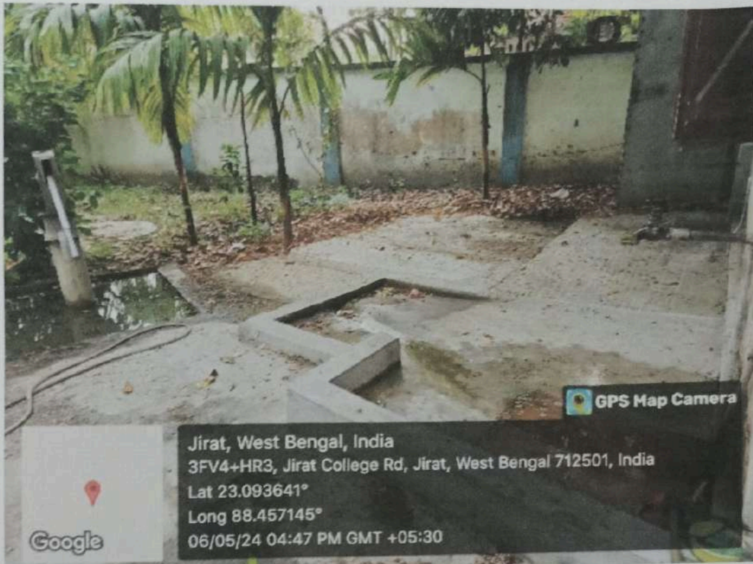
Vertical Filter Chamber With Silt Chamber (1)
