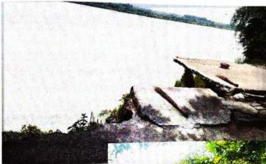
RIVER BANK EROSION SITE
