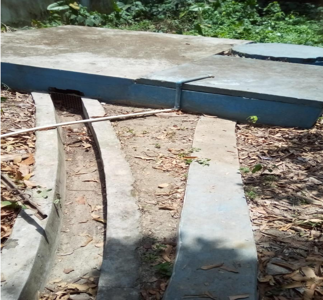
Pipe Line Connection for Rain Water Harvesting in College Campus and pipelines come directly from the rooftop of Main Building of this college
